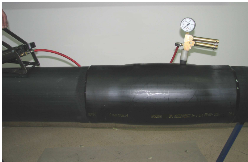
Photo No. 33 Control pressure gauge mounting
